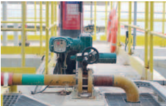
Extreme conditions: Heat combined with salty maritime air. SG part-turn actuators with AUMA MATIC within an industrial plant in Qatar.
