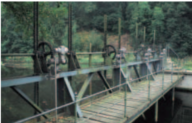
SA/GK multi-turn combinations with AUMA MATIC actuator controls integrated in a historical weir in East Germany.
