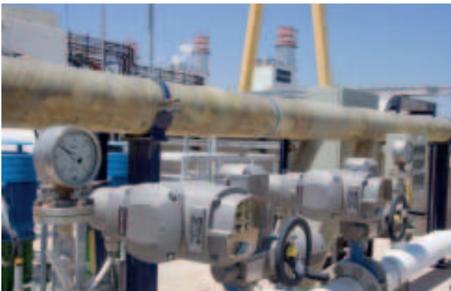
SG part-turn actuators with AUMA MATIC within a combined cycle power plant in Spain.
