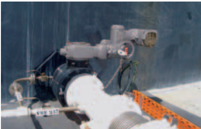
Explosion-proof SAE/C/GS multi-turn/part-turn actuator combinations with AUMA MATIC mounted on a butterfly valve within a tank farm in the Azores.
