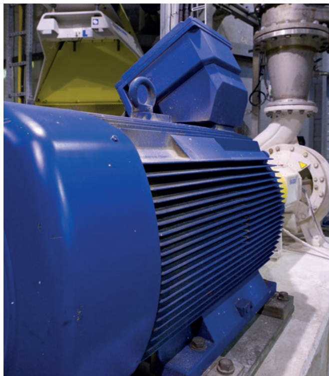
Pump drives in a paper machine
